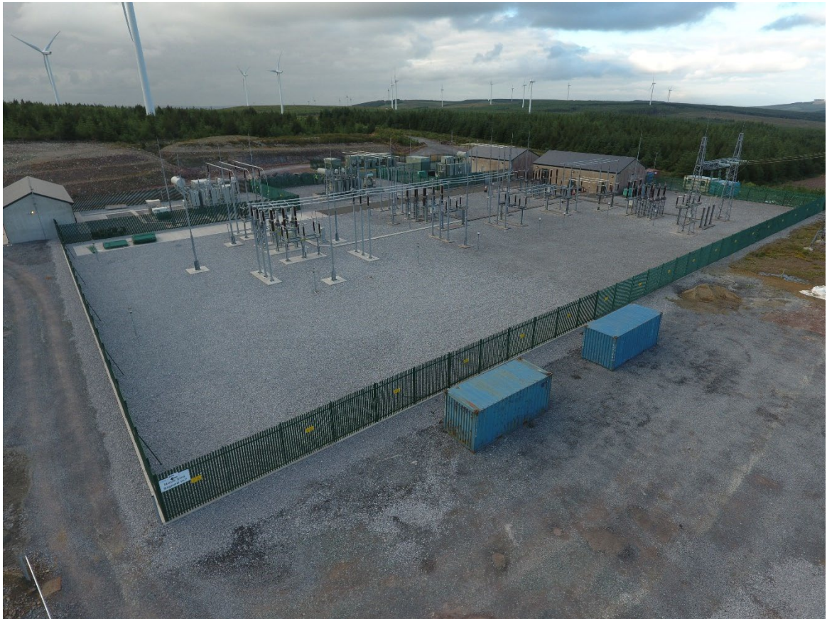
Photo 4.3 Typical 132kV substation compound
