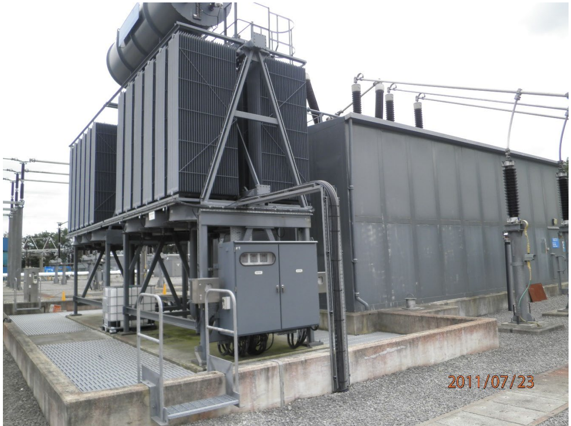
Photo 4.2 Typical (large 400kV) power transformer
